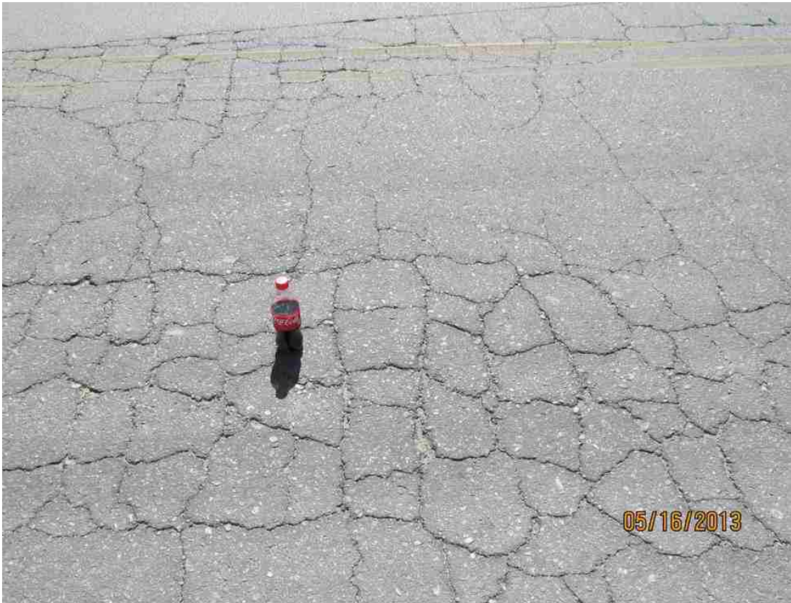
Figure 3. Pavement alligator cracking
