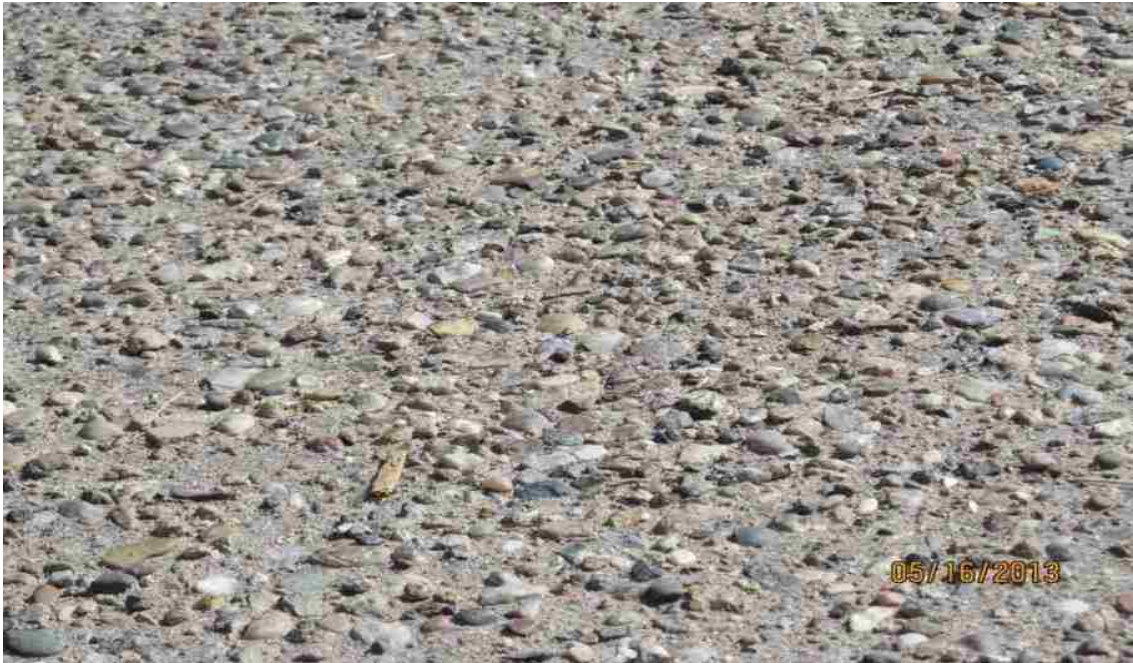
Figure 1. Raveling and weathering of flexible pavement
