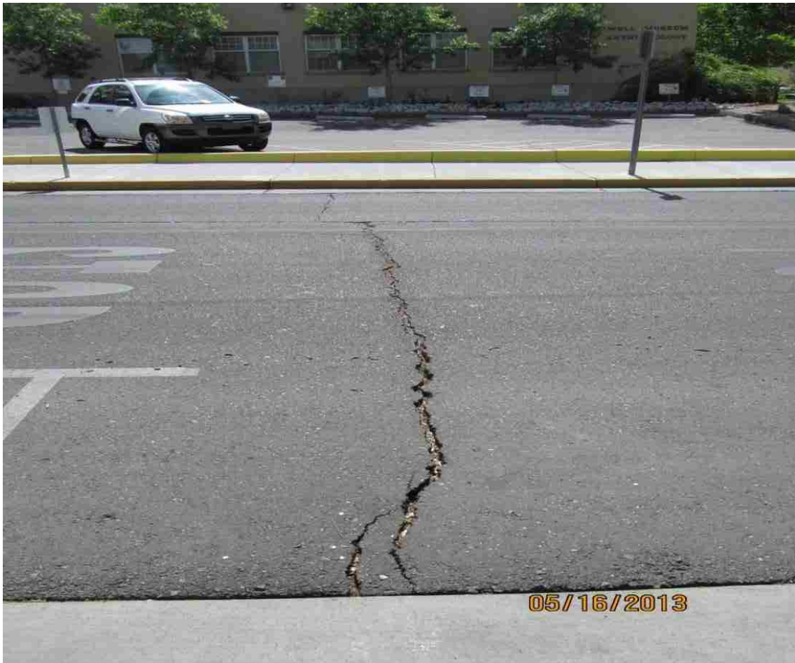
Figure 4. Transverse pavement cracking
