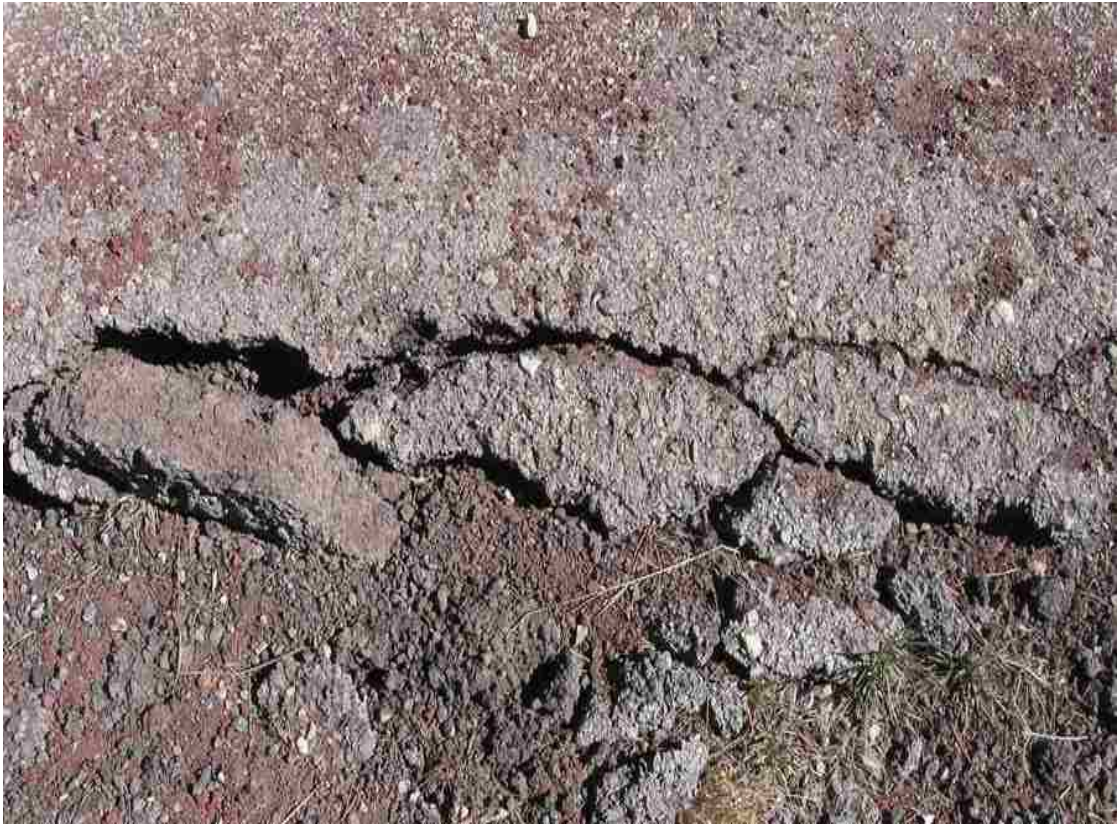
Figure 5. Edge cracking of flexible pavement
