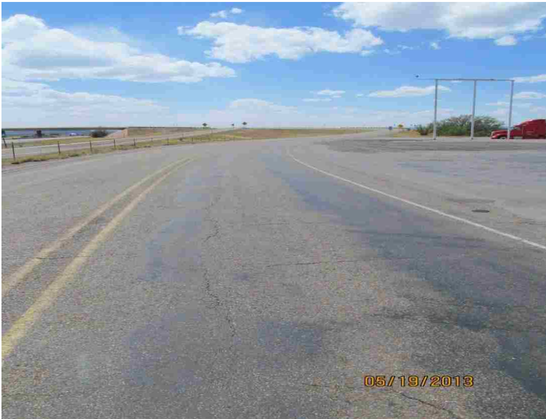
Figure 2. Pavement asphalt bleeding
